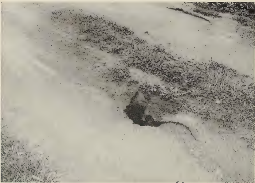
FIG. B—Gopher hole caved in and water-filled in a wheel track of a roadway during a two-day rain. By next day this hole was completely filled with dirt washed in, and afterwards only a slight trace of it could be detected. Photographed on December 14, 1934.
